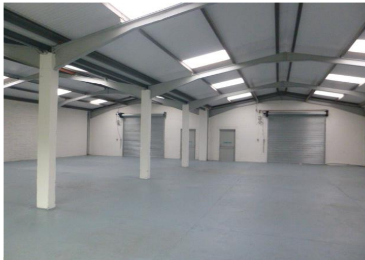
Fig 1. This building has no EPC, it looks new, there are no fixed services, it could be shell and core
